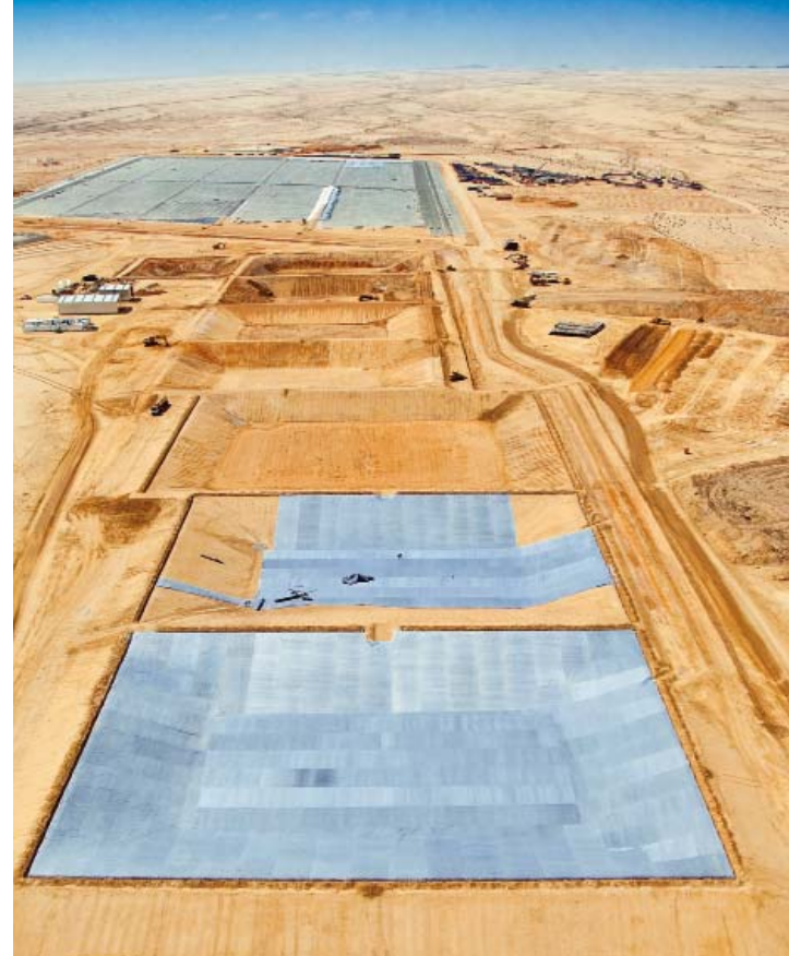
Pads on a uranium mine showing the necessity for accurate levelling over an extensive area, made easy with the Trimble systems.
